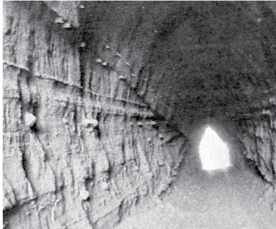
Photo shows the top of inside of the tunnel. Note wire netting "nailed" to the top to stop rocks falling on vehicles passing below. Note the width of the road edge and it is not level. "Heart in your mouth" stuff if you meet a large truck. This is part of a Carrington Rd to Mt. Messenger walk undertaken by a 73 year old completing a 689 km hiking trip across the North Island to Cape Egmont.
